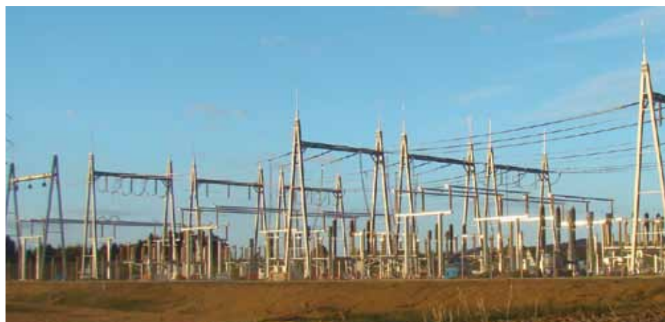
Transpower's Drury substation
